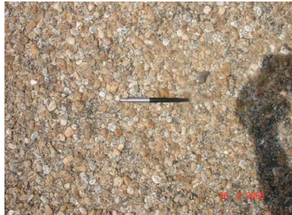
The double Otta seal surfacing constructed from screened quartzitic gravel obtained from adjacent to the road alignment.
